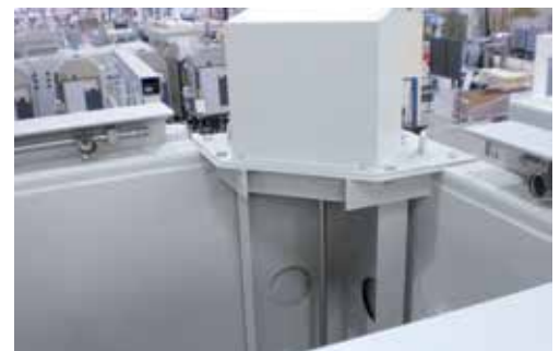
Protective gas supply as fire protection
