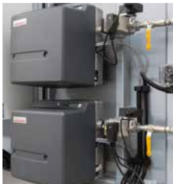
Gas burners for furnace heating and thermal afterburner
