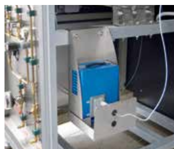
Acid pump for nitric acid
