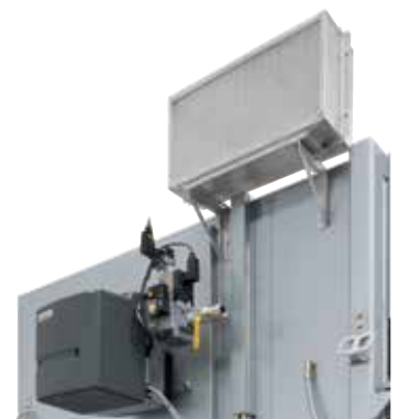
Direct gas-firing at a chamber dryer
