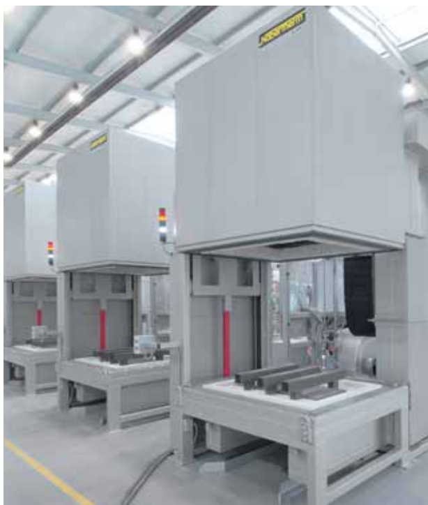
Production plant, consisting of 3 top hat furnaces HAS 1560/95S with sealed housing for operation with nitrogen. Including air/gas heat exchanger for reduced cooling times
