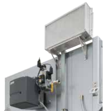
Direct gas-firing at a chamber dryer
