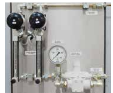
Gas supply system for non-flammable protective or reaction gas
