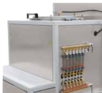
Cooling water distribution
