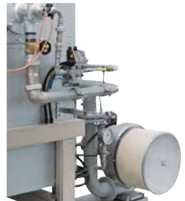
Gas line for natural gas
