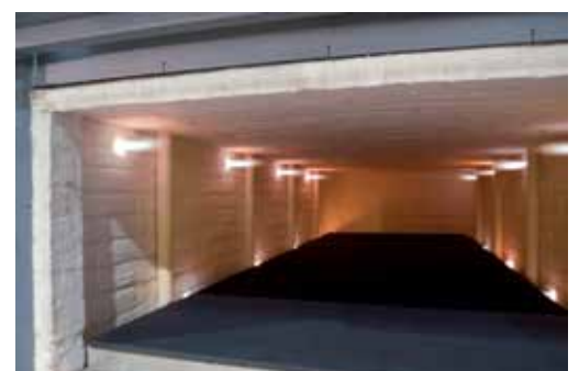
Furnace chamber with eight high-speed burners
