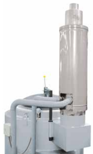
Heat exchanger in the exhaust gas duct
