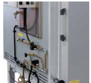
Gas lines and thermocouple at the chamber kiln
