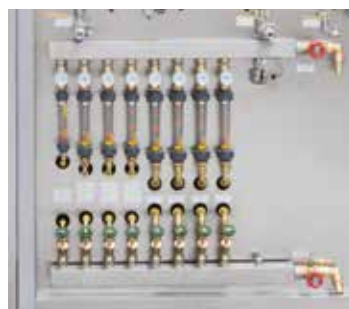
Cooling water distribution
